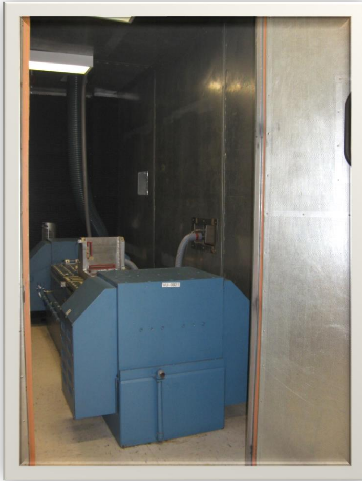
Control Room Open
